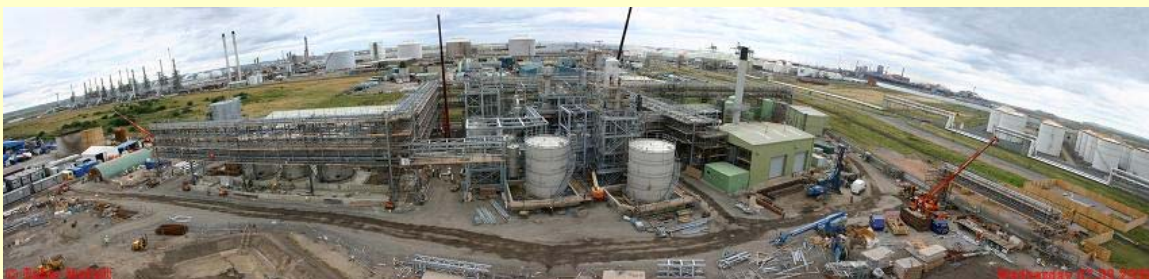
Figure 27: View of Biodiesel Production Plant in Teesside, UK
