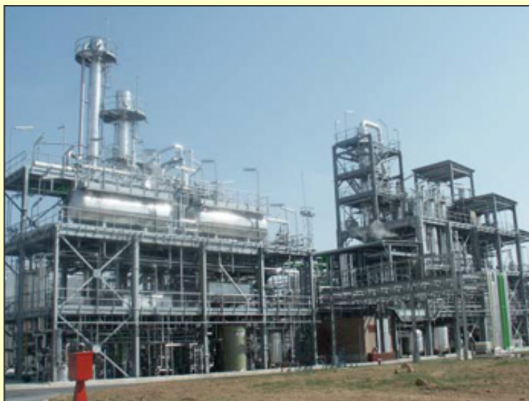
Figure 31: Overall View of the Biodiesel Processing Unit
