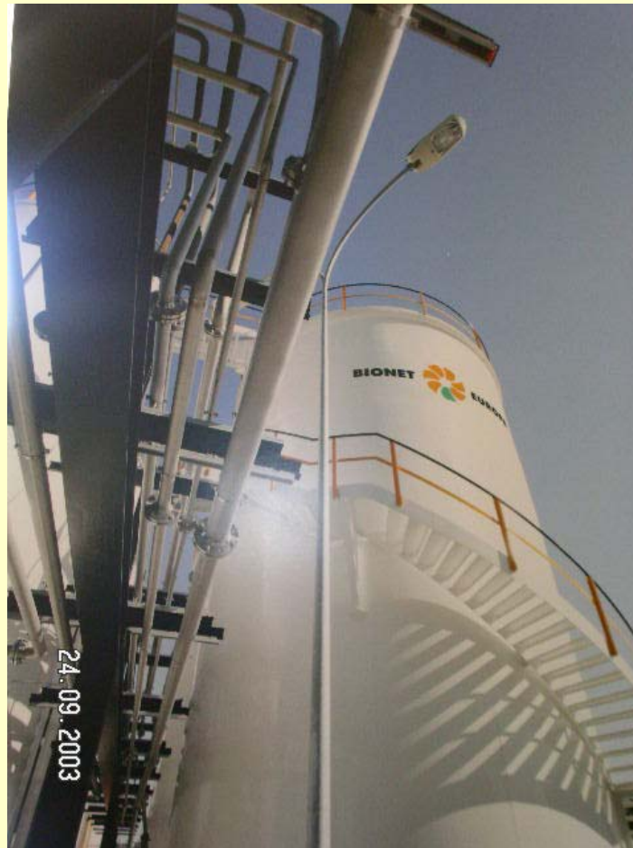
Figure 6: Tank farm of the Bionet Biodiesel plant
